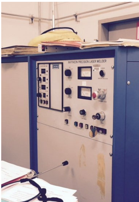
Large external power supply for laser welding machine. ECCN: 2B999.c
